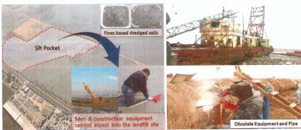
Fig. 1. Problems in Dredging and Reclamation (Saemanguem Industrial Complex Reclamation Site)
